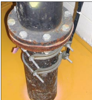
This 4-inch riser should be surrounded by an 8-inch diameter hole.
